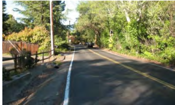
Figure 3-5 Missing Sidewalk in Trotter/ South Walnut Creek
